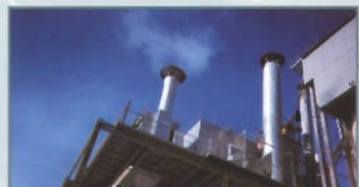
Filtering installation for Drying sepiolite SEPIOLSA (GUADALAJARA-SPAIN)
