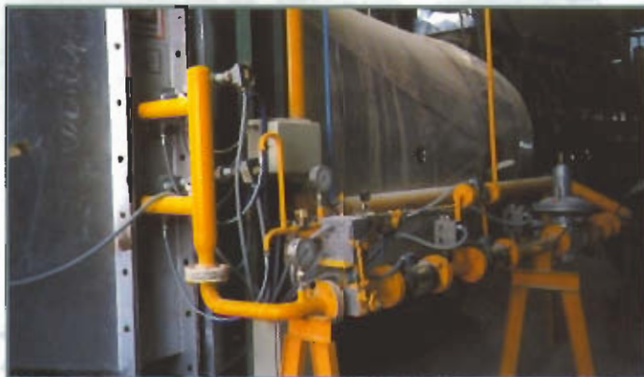
Combustion Chamber by air vein INSTALLATION for GUBRE-TURKEY
