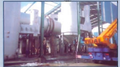
Installation of Drying waste material for Incineration furnace SOGAMA (GALICIA-SPAIN)
