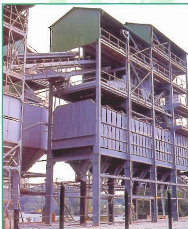
Criblage de charbon - FRANCE
