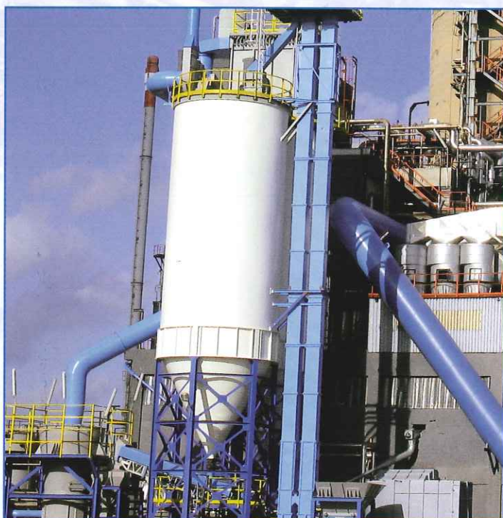
Silos and bucket elevators: FERTIAL (Annaba, Algeria) Dolomite.
