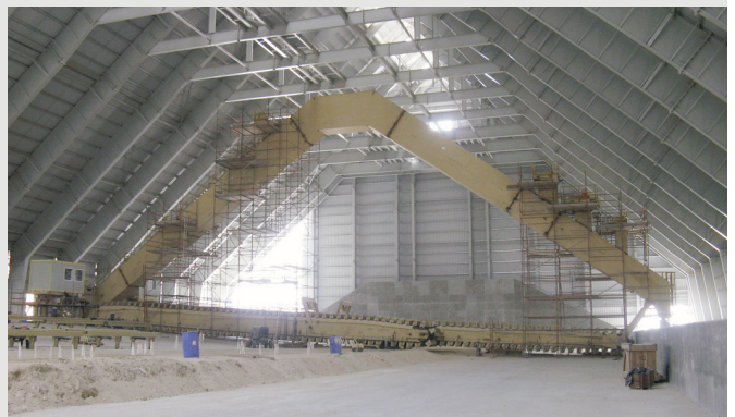
Portal scraper at the indoor storage park for phosphate and additives of 21,300 m 2 and 160,000 T for the whole chemical complex of Ras Az Zawr. Customer: MA'ADEN/WORLEY PARSONS – Engineering: LITWIN.
