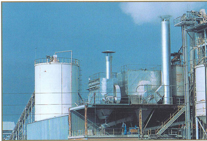
Dedusting Plant-Cogeneration Fluid Bed-Sepiolsa SPAIN.
