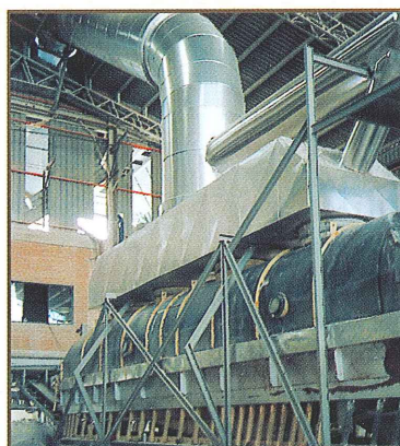
Vibrating Fluid Bed cogeneration-clays
