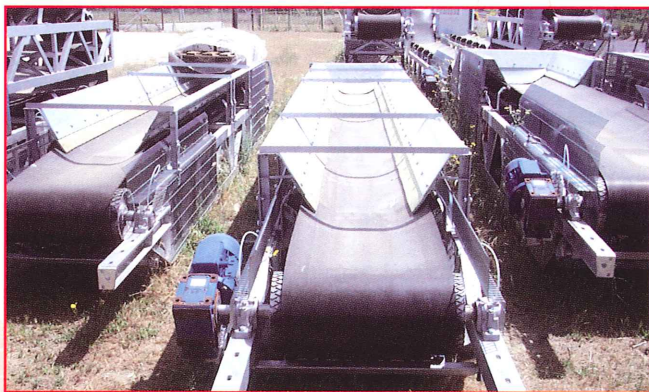
Conveyor belts, CAN. Fertil (Arzew, Algeria).
