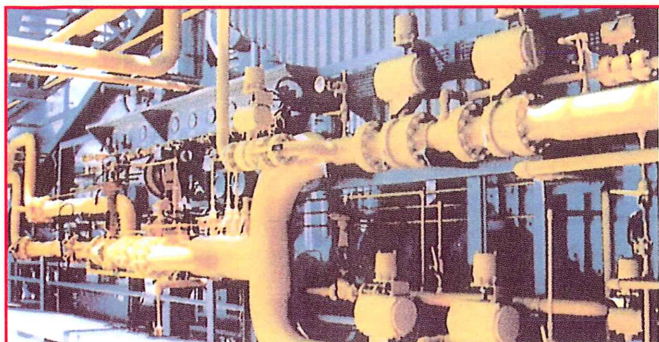
2 hot gas generators, 2 x 30,000 Th/h for TSP, PK. NPK dryers. Asmidal Annaba (Algeria).
