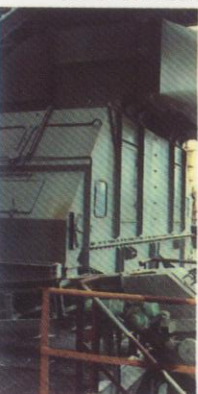
Urea prills tower cooling Enfersa Cartagena (Spain)
