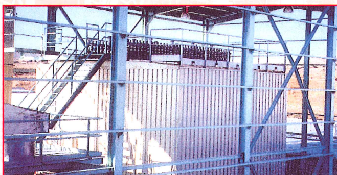
Bag filter jet 160-2L-10, Dryer + Granulator + Cooler of Fertilizer, NPK. Inabonos (Spain).
