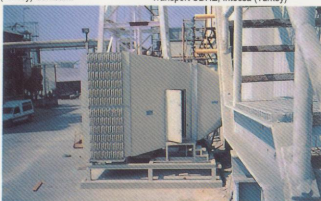
NPK cooling 1,200,000 frig/h. Fertiberia Huelva Plant. (Spain).
