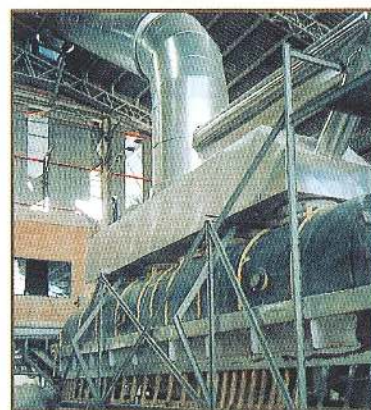
Vibrating Fluid Bed cogeneration-clays
